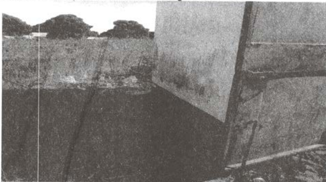
Picture 1: The only functional Toilet at Ndungu Kebbeh Lumo
