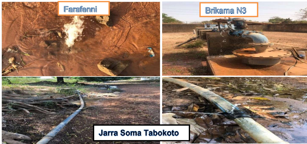
Picture 3: Burst pipes in Farafenni (top) and Mansakonko (down)
