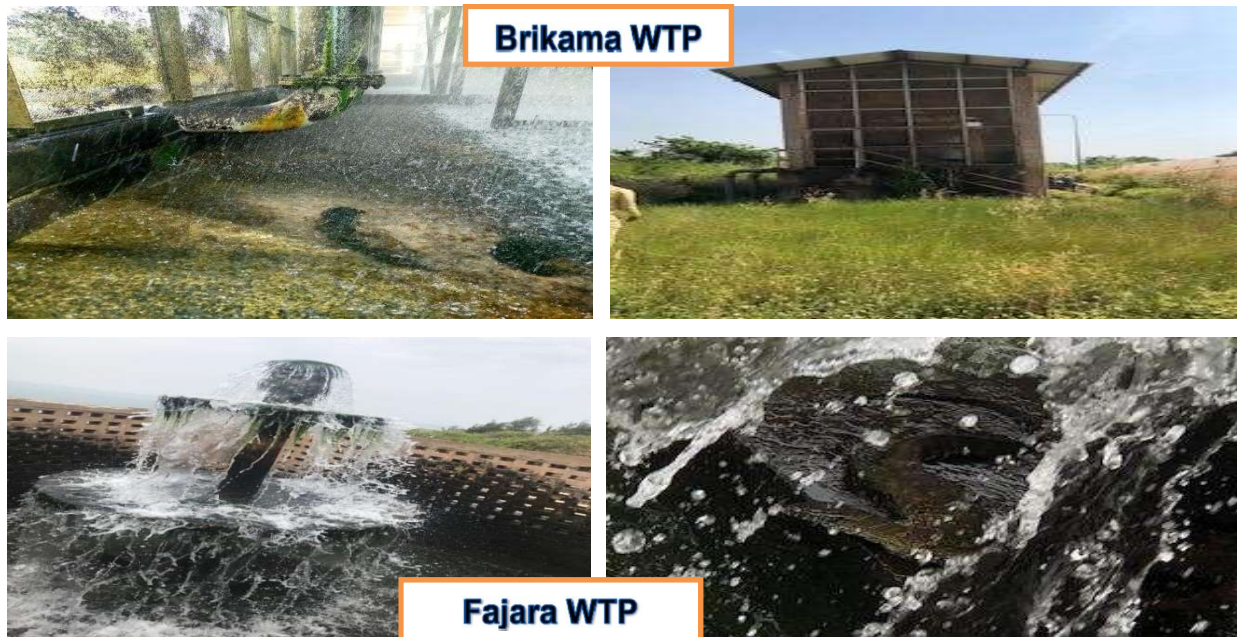
Picture 9: Condition of the aerator at Brikama Water Treatment Plant (Top left and top Right) and aerator condition at Fajara Water Treatment Plant showing a reptile (Monitor Lizard) inside the aerator.
