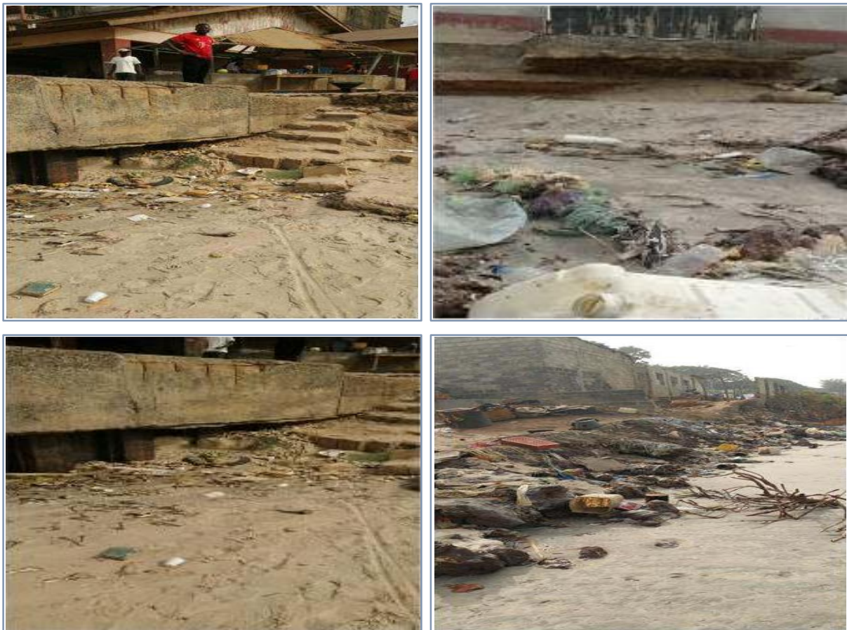
Picture 11: Showing dilapidating structures at the Bakau CFC
