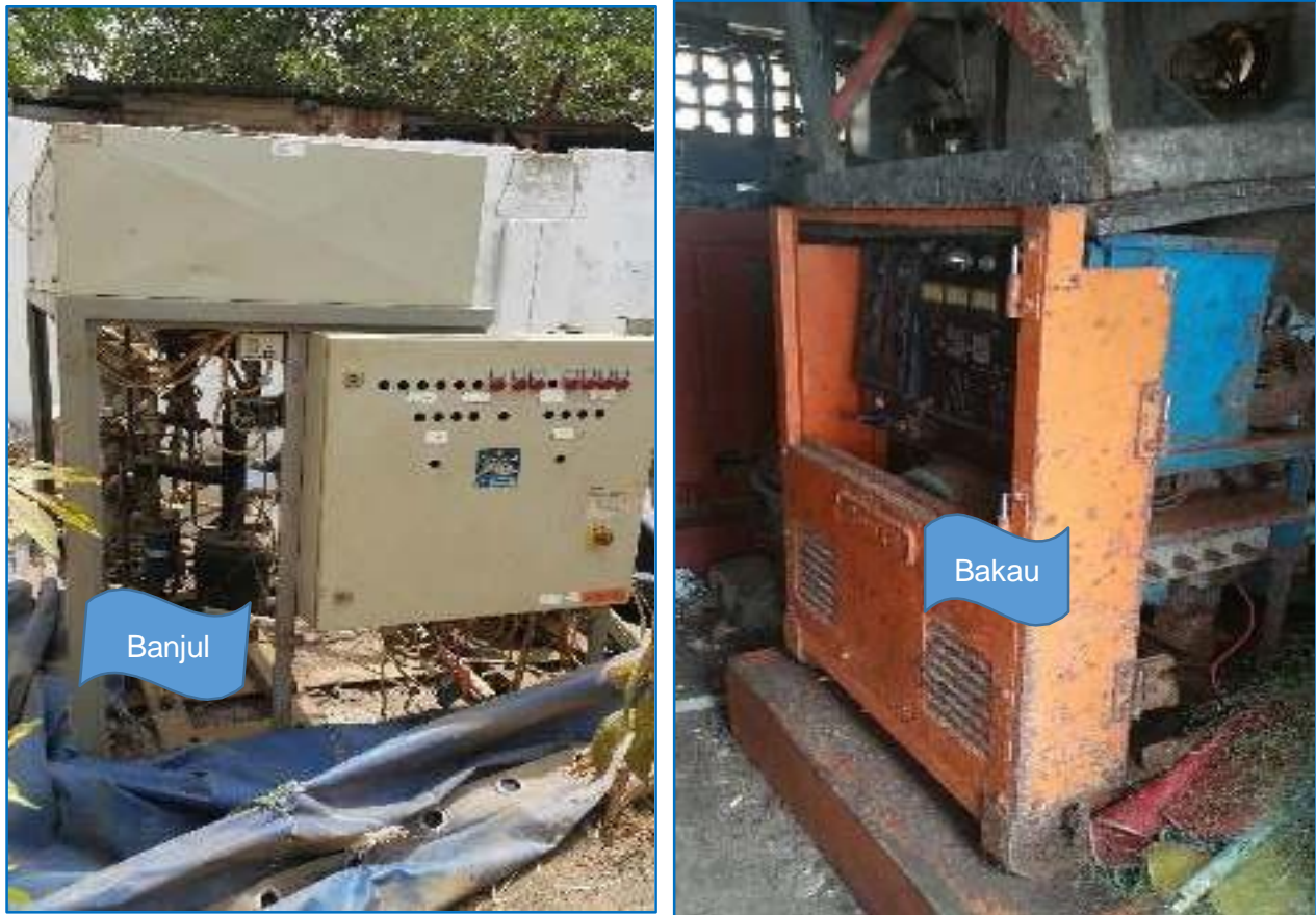
Picture 10: showing broken down or dilapidated ice plant machines in the CFCs
